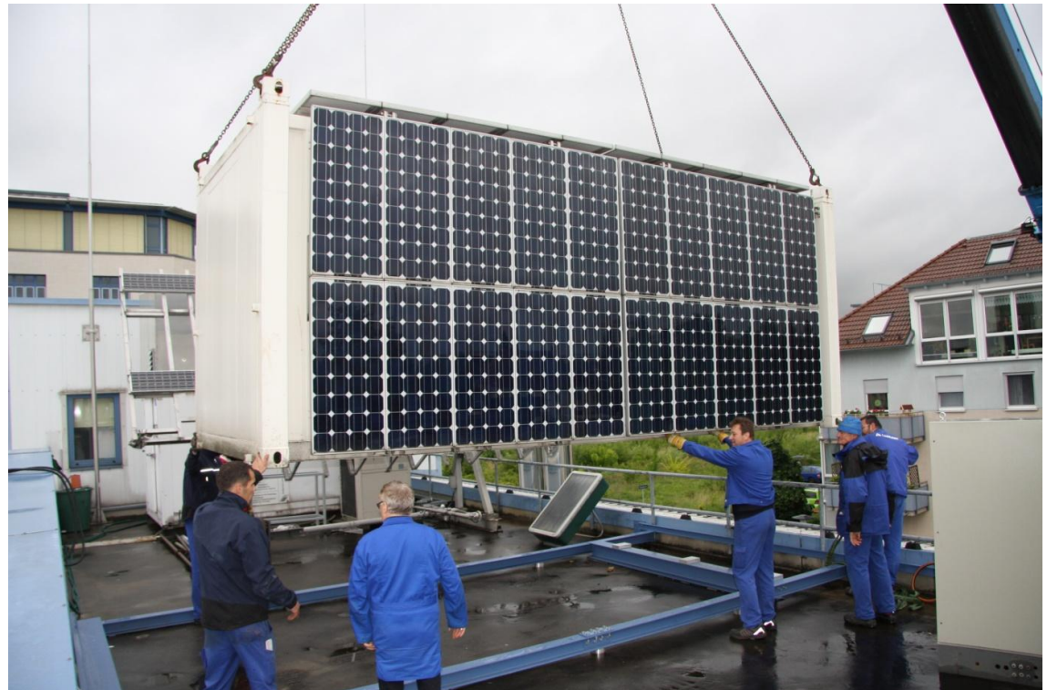
Transport of a cooling container ready for operation at ILK Dresden
