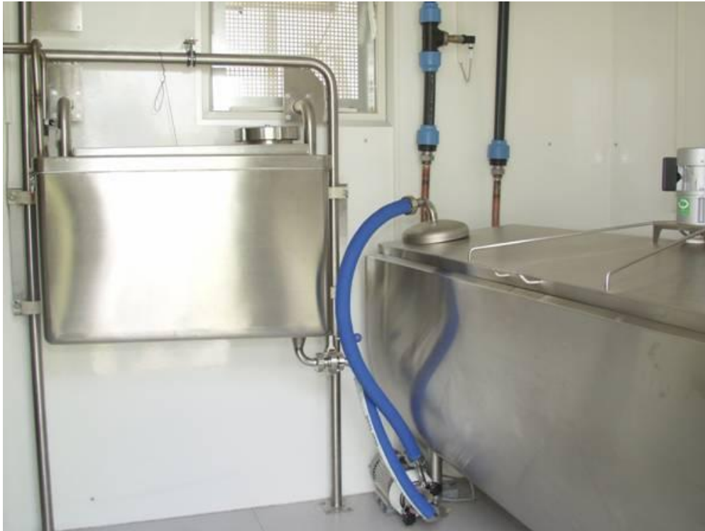
System for cooling and cold storage of milk
